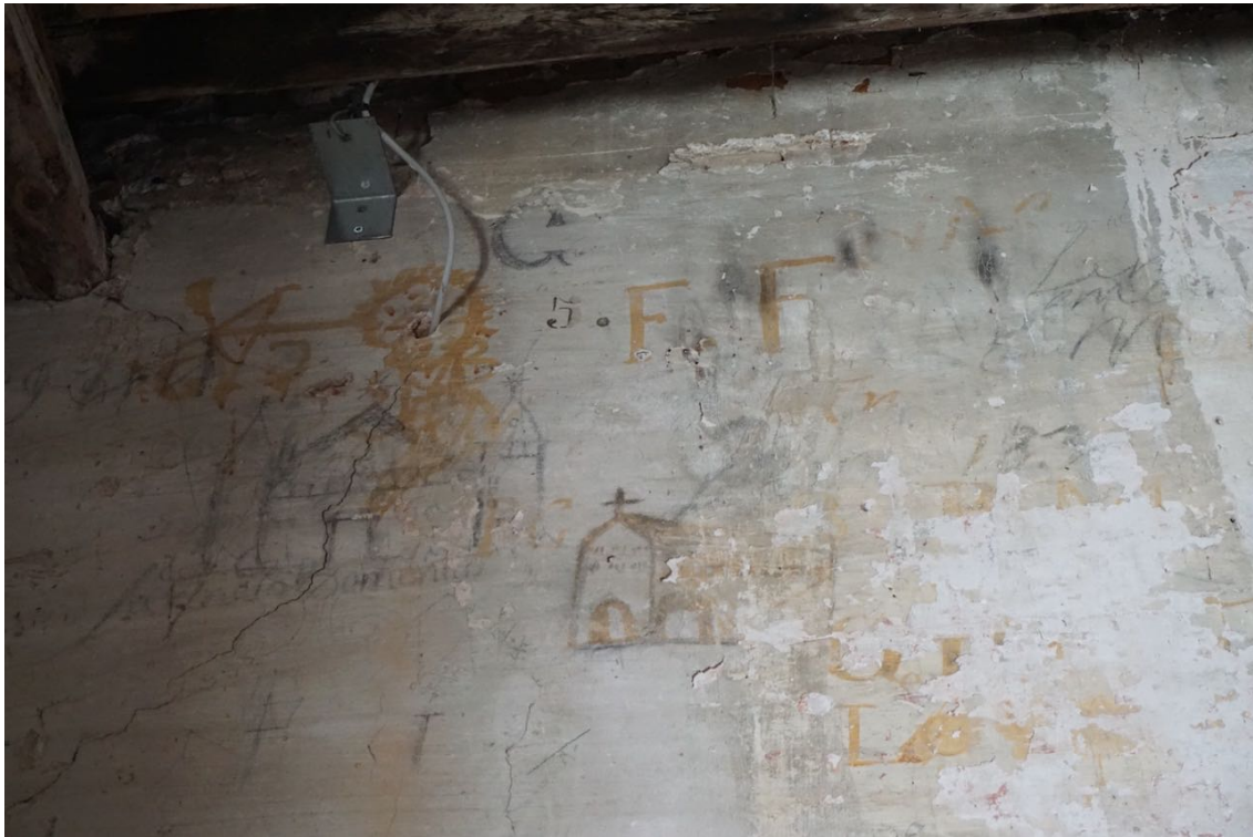
Figure 3.45: Graffito damaged by structural additions at the Lazzaretto Vecchio
