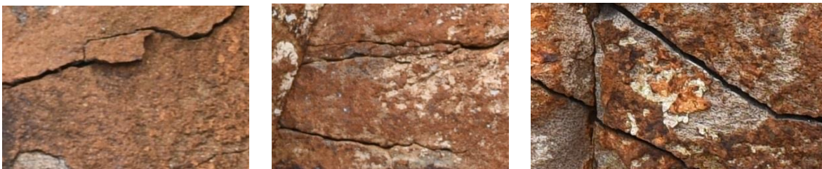
Figure 4-12: Examples of staining of weathered basalt
