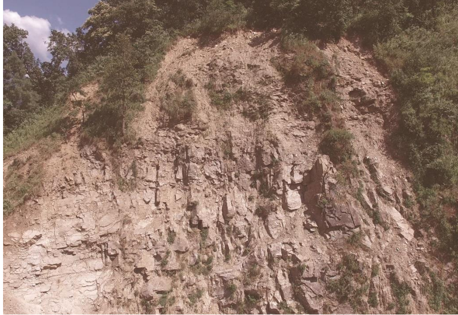
Figure 3-22: Photo of landslide back-scarp revealing weathering profile
