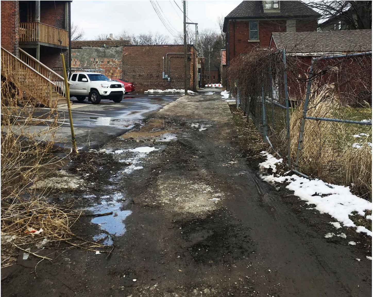
Image 24: In the West Village, Alleys are used as important neighborhood connectors to residences. As seen from the photo, the state of the paving material is in poor condition. (Source: Authors)
