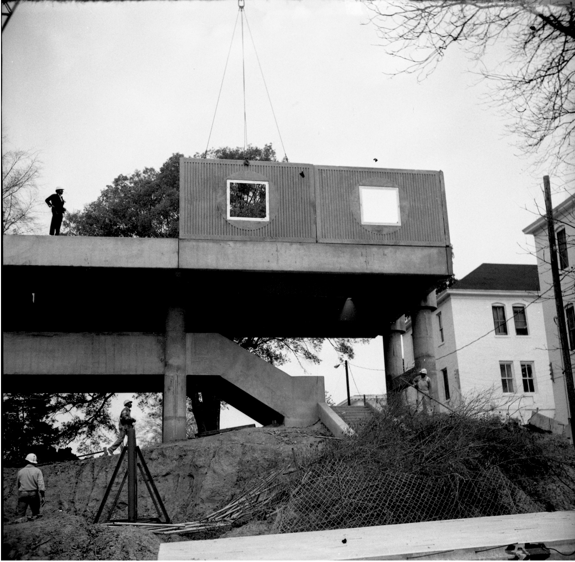
Figure 2.14 Tougaloo College dormitory construction photograph showing positioning of wall panel atop first residential floor. Box 5, GBA records, BHL.
