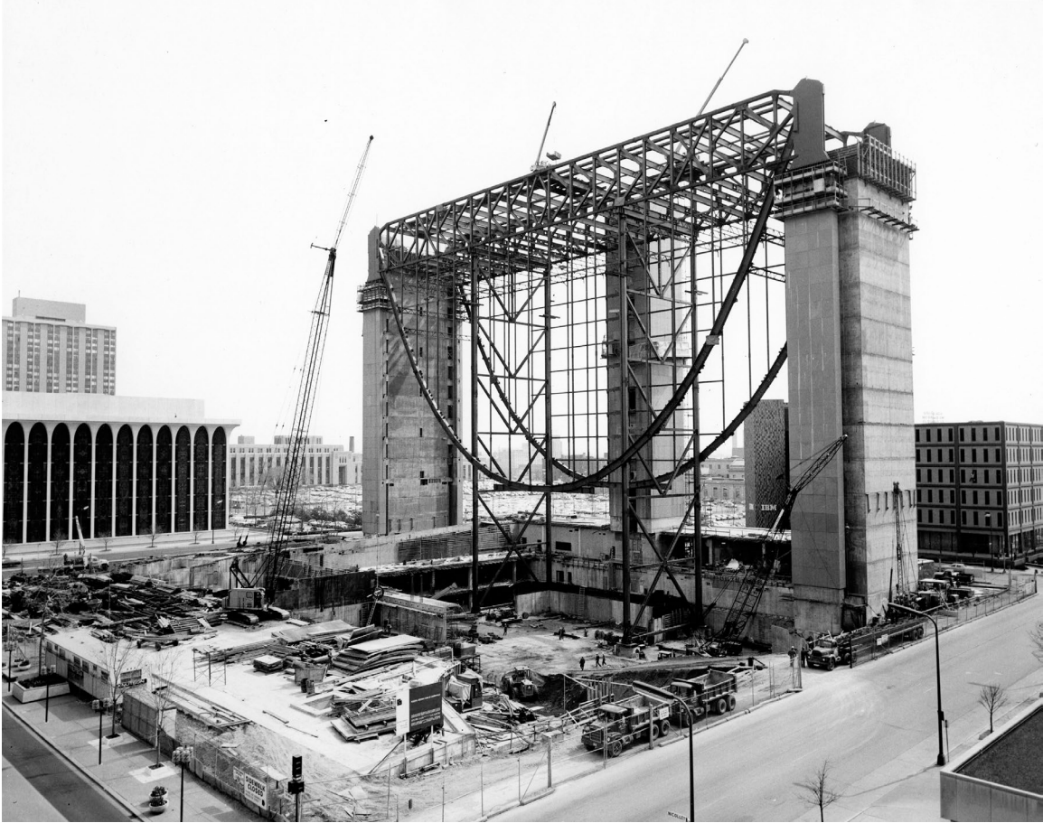
Figure 3.24 FRBM construction progress photographs showing preparation of steel suspension structure, April 16, 1971. Seen at left is the Northwestern National Life Building by Minoru Yamasaki and Associates, completed in 1965. Black and white print, 8.75 x 10.75 inches. Photograph by Schwang Studio. Box 21, GBA records, BHL.
