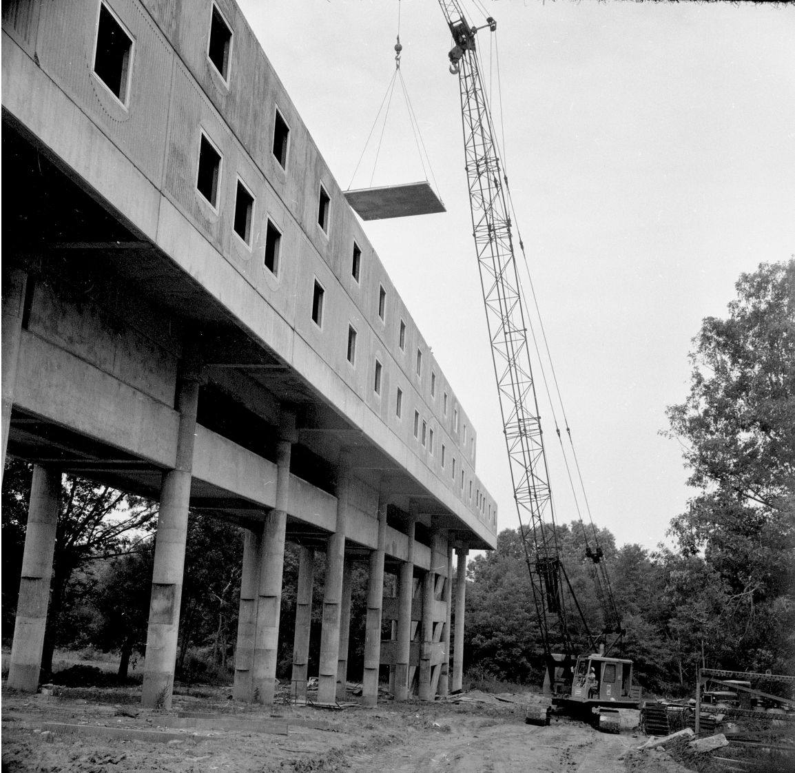
Figure 2.43 Tougaloo College dormitory construction photograph showing positioning of roof panel atop second residential floor. The access walkway is below the first dormitory floor between the structural columns. Box 5, GBA records, BHL.
