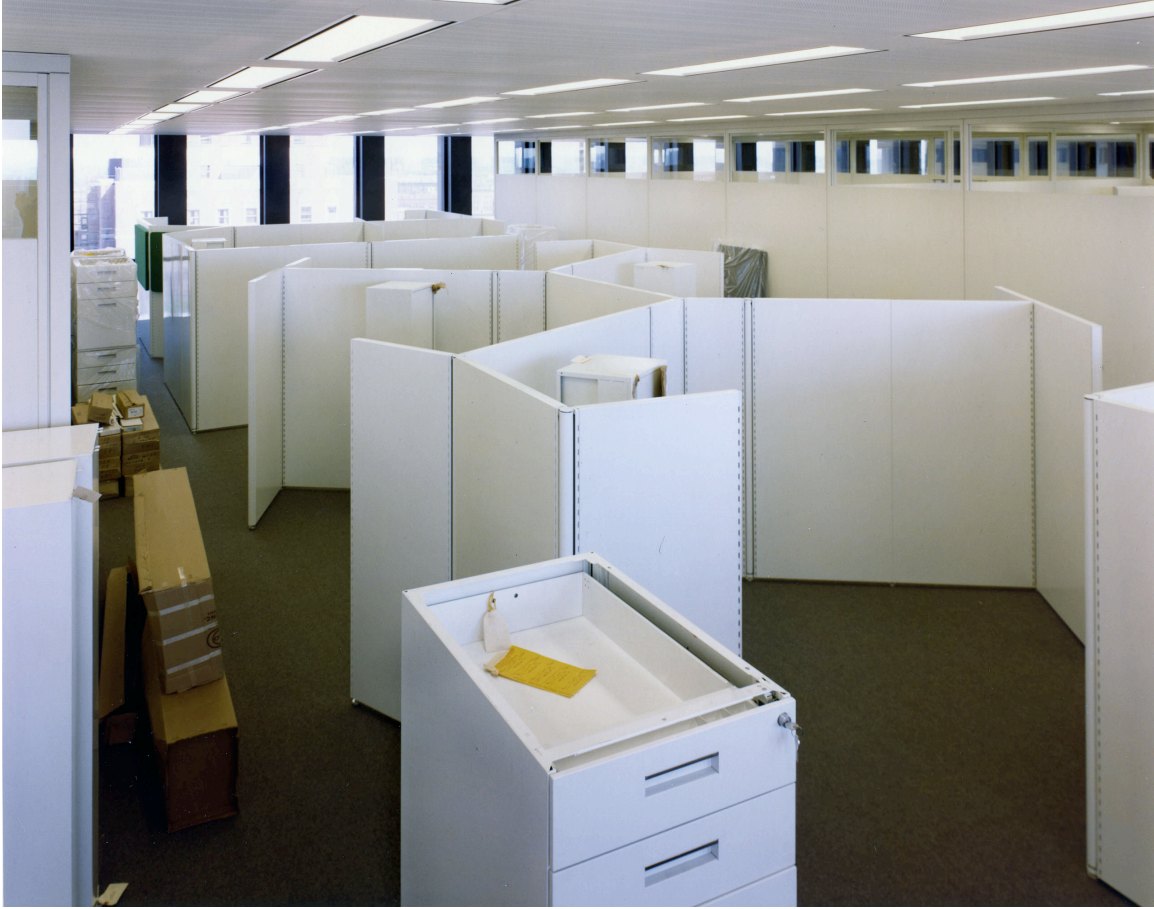
Figure 3.42 Installation of workstation systems in FRBM. Photographer unknown. Box 19, GBA records, BHL.
