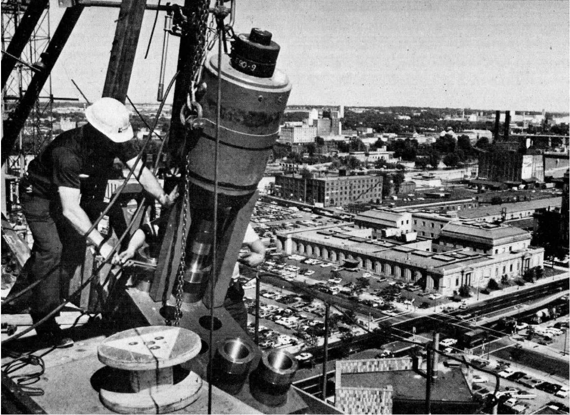
Figure 3.23 A steelworker tensions one of the eight suspension cables that support the FRBM office tower, April 1971. From: Federal Reserve Bank Ninth District, "Cablegram: Fact Sheet/The New Federal Reserve Bank," September 7, 1973. Box 17, GBA records, BHL.
