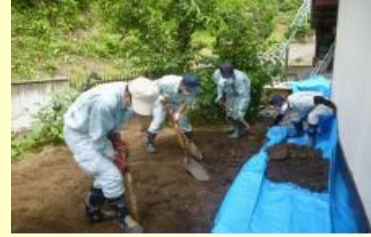
Removal of soil surface cm by cm with hand shovels & carrying out of removed soil to deposition site
