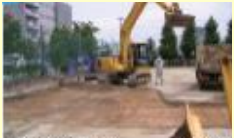
Removal of surface soil of school ground with heavy machine and burying in a pit bored in the ground
