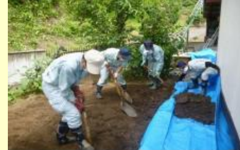
Removal of soil surface cm by cm with hand shovels & carrying out of removed soil to deposition site
