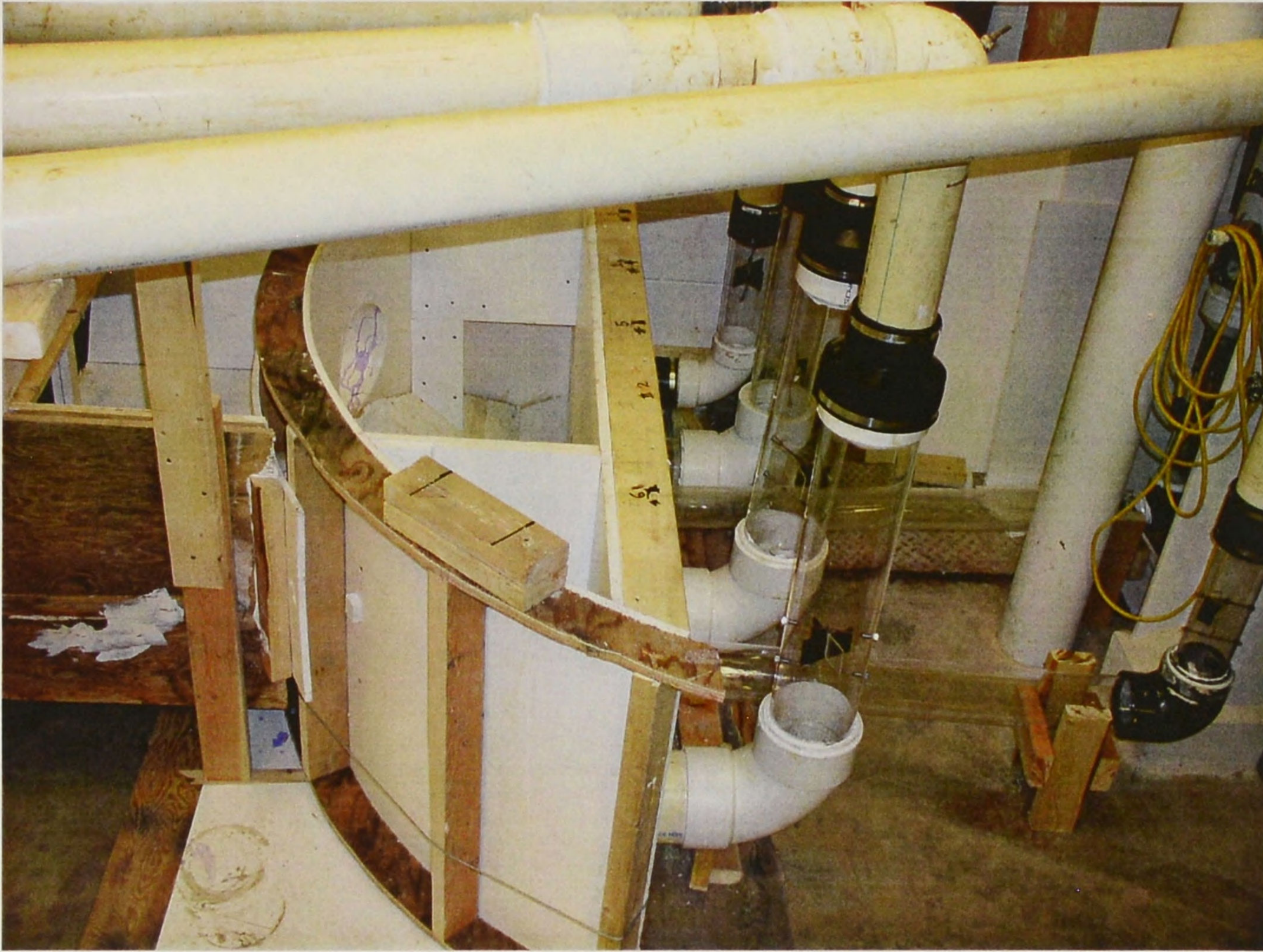
Figure 3. Wet Well and Pump Intakes.
