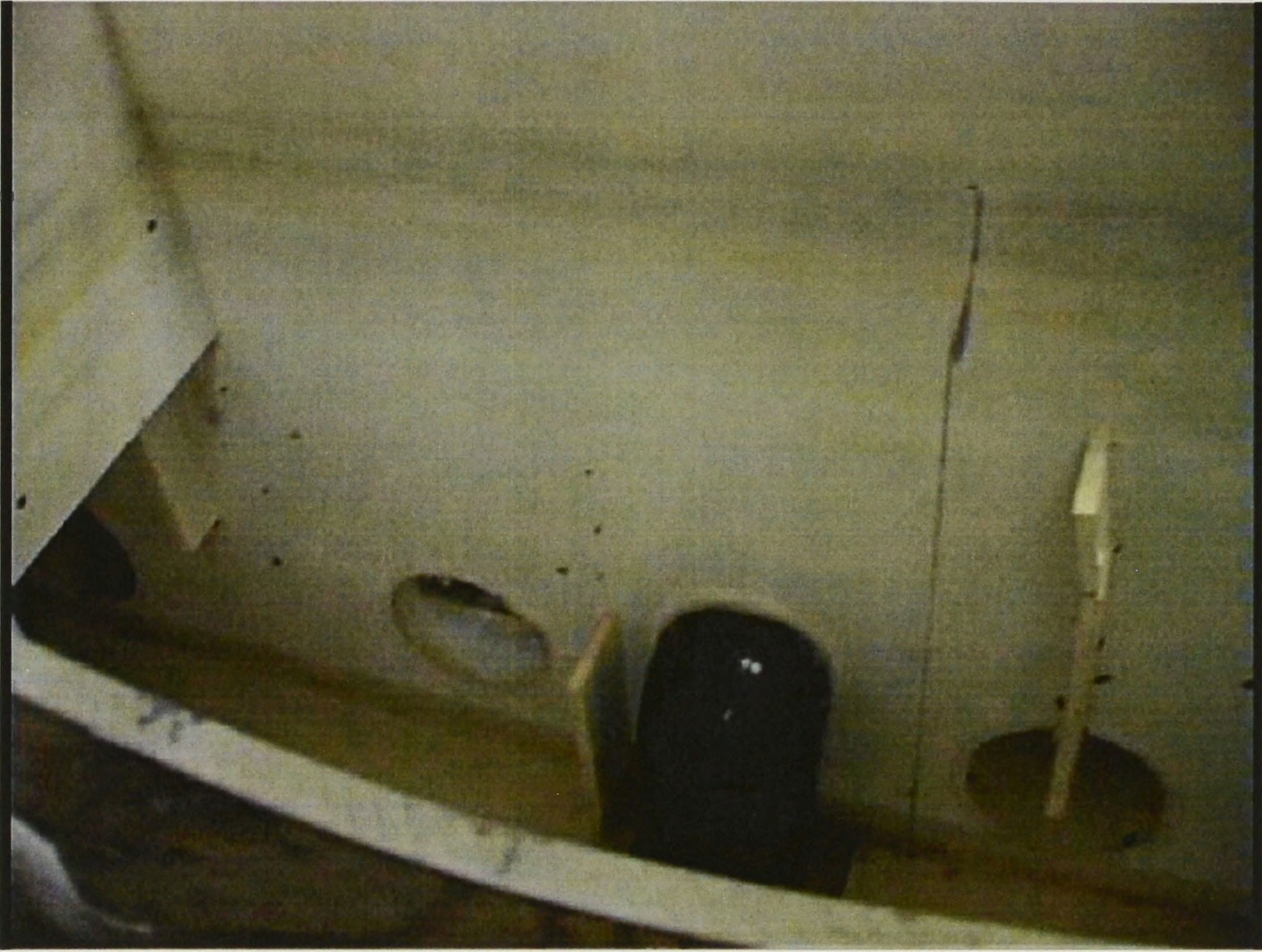
Figure 14. Plates located near intakes of pumps #4, #3 and #5.
