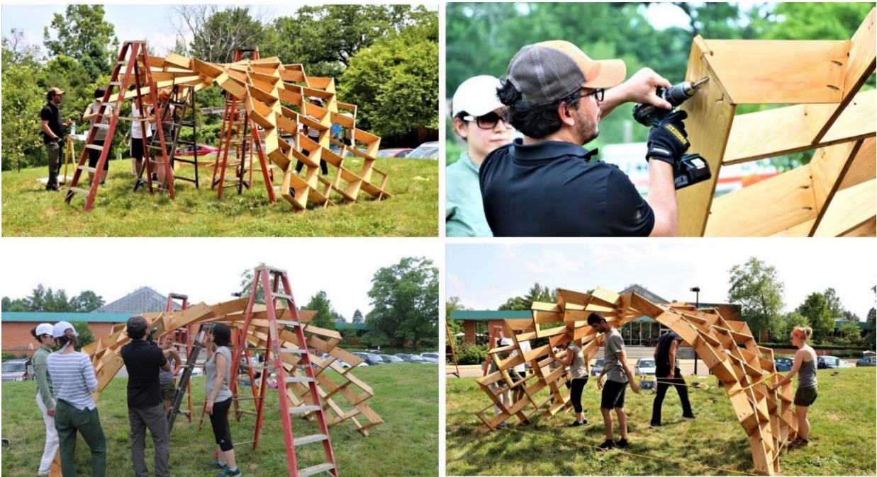
Figure 231_ a) Erecting the arch from three pre-assembled pieces using two support ladders. b) assembling the connecting pieces using screws c) assembling the last pre-assembled piece of the arch. d) supporting the arch using bracing ropes.
