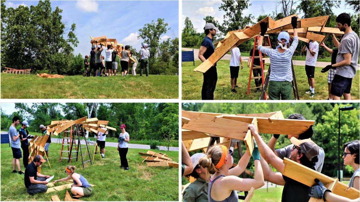
Figure 230_ Moving the preassembled pieces of the arch to the site location for setup.
