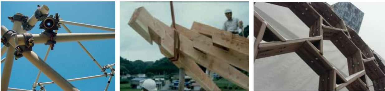
Figure 40_ Fabrication of reciprocal connections. From the left: clamped connection, notched connection, T-joint connection.
