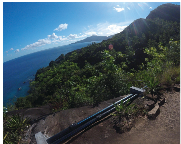
Utility pipes along a hiking trail in Anse Major.
