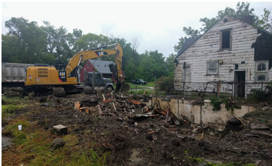
Figure 2 A typical demolition site with excavated basement in front of an excavator and waste hauler. Photo by author.
