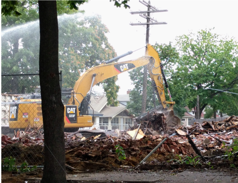
Figure 13 Following 'knock down,' an operator uses a grapple-bucket excavator to 'load out' a small commercial building. Out of the frame, a laborer uses a firehose to direct water onto the bucket. Photo by author.
