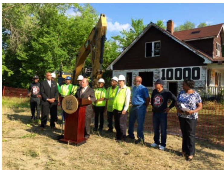
Figure 4 Detroit Land Bank Authority, 10,000th demolition celebration July 19, 2016. Screen capture from Detroit Mayor's Office Facebook Live, downloaded September 15, 2016
