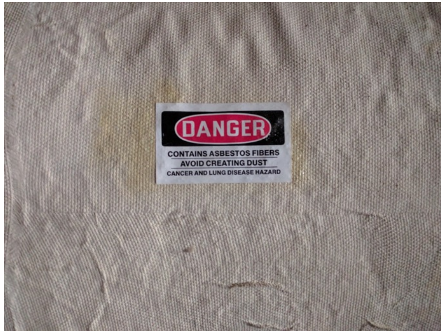
Figure 16 Asbestos hazard in place. Photo by author.
