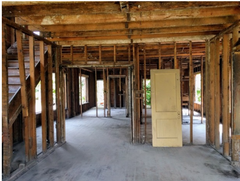
Figure 19 After abatement. These were previously plaster walls and ceilings. Photo by author.
