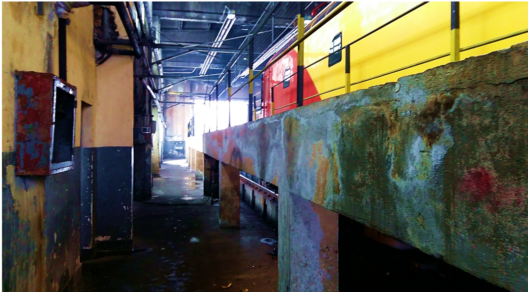
Illustration 21. Degradation in the square shed.
