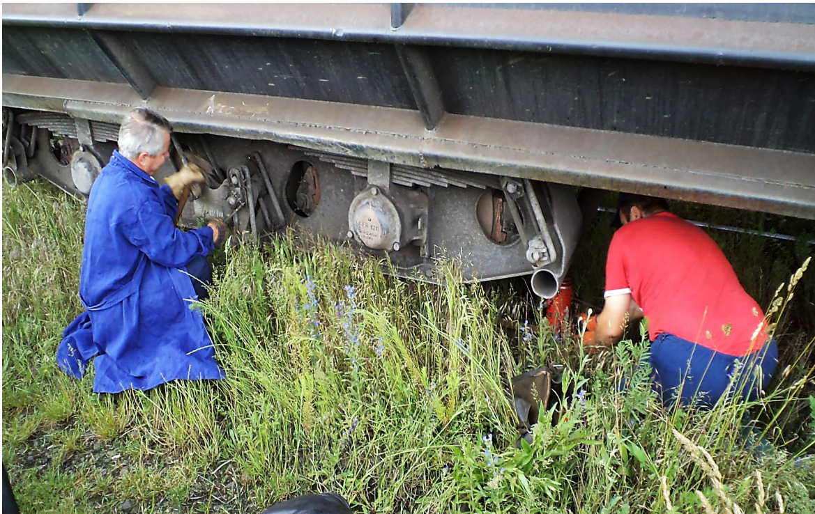
Illustration 27. Repairing the spring leaf. The red instrument to the right is the defective jack.
