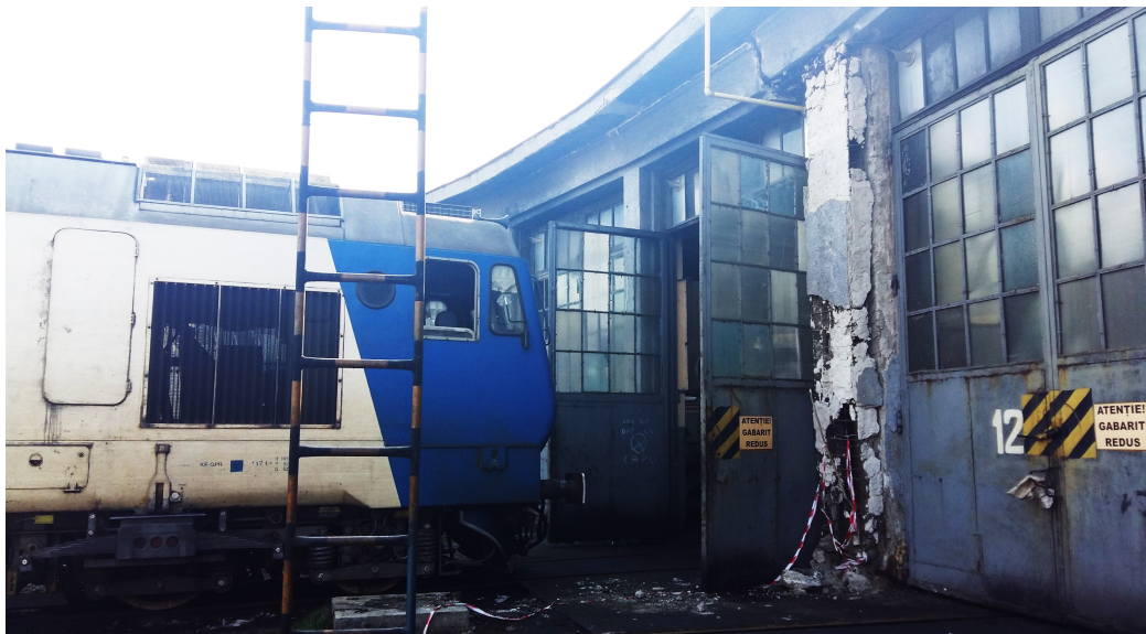
Illustration 19. Eroded supporting pillar at the roundhouse.
