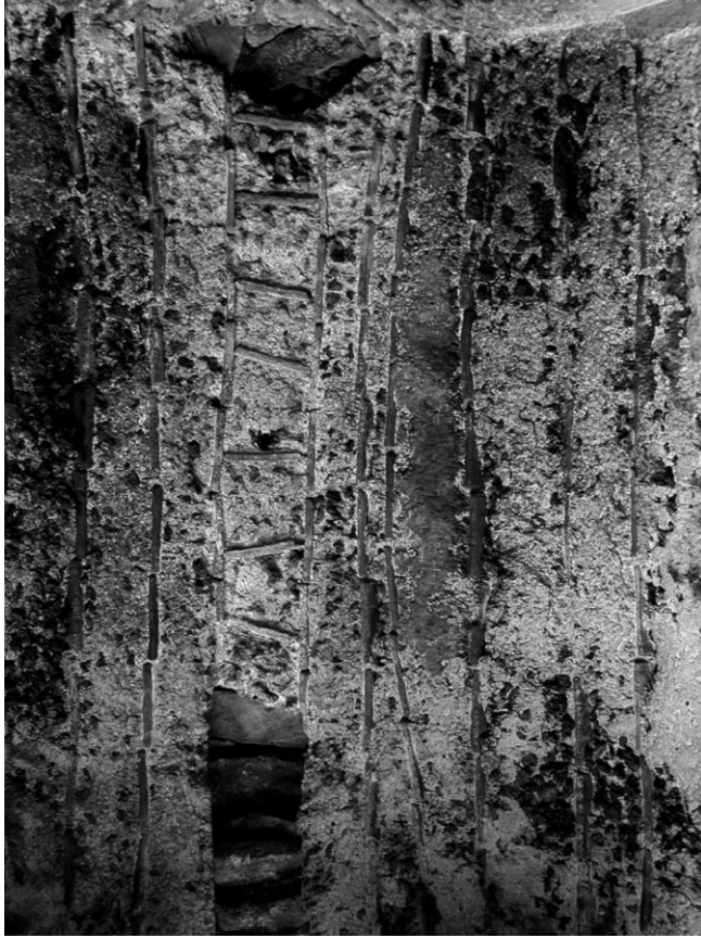
Figure 159: View looking up at the vaulting in the frigidarium of the baths at Selaema (modern Salim), showing mortared rubble with scoria as caementa set between vertically placed bricks (Fournet 2010, fig 12).
