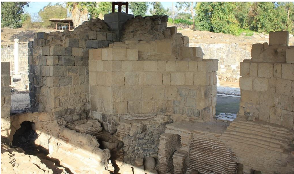
Figure 92: Interior view of the Western Bath at Scythopolis (modern Bet She'an), showing use of basalt and limestone ashlar masonry in a reconstructed wall (only the bottom two courses are original) (photo by author).
