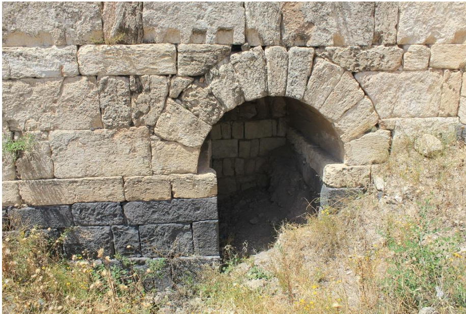
Figure 86: Close-up view of the masonry of the Byzantine Baths at Gadara (modern Umm Qais), showing use of basalt ashlars under limestone ashlars (photo by author).
