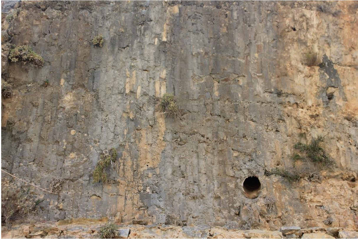
Figure 147: Close-up view of vaulting of Bath III 2 B at Anemurium, showing the impressions of vertically set bricks (now fallen away) in the mortared rubble packing (photo by author).
