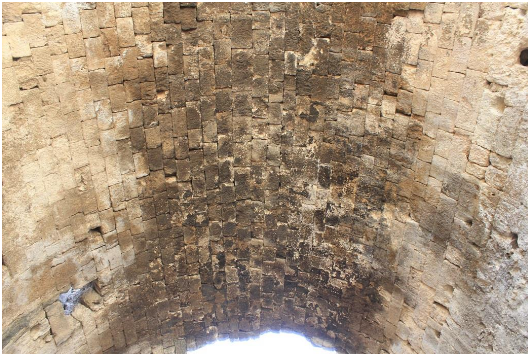
Figure 169: View looking up at the intact ashlar vaulting of the East Baths at Gerasa (modern Jerash) (photo by author).
