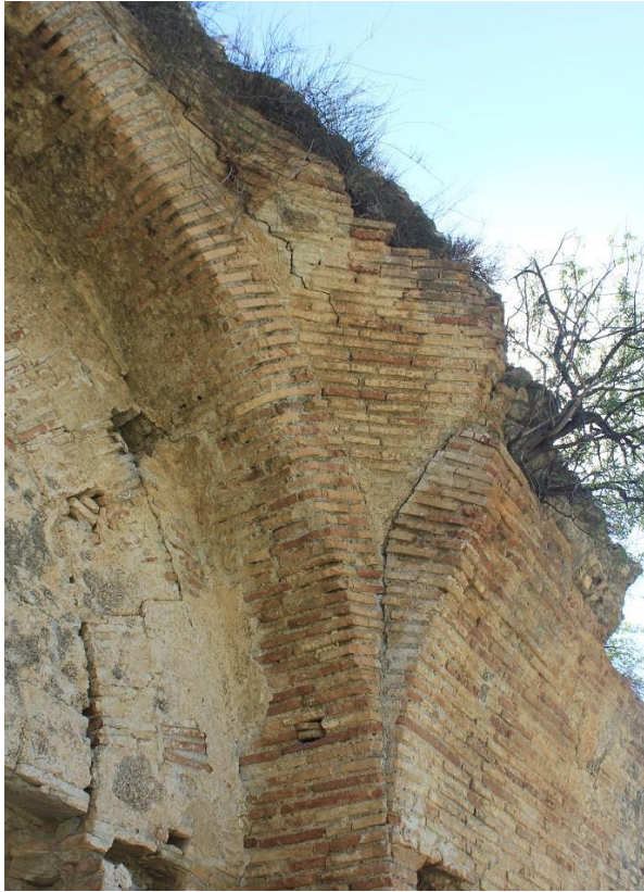
Figure 151: Close-up view of pendentive in the Northern Baths at Anazarbos, showing use of radially set bricks in vaulting (photo by author).
