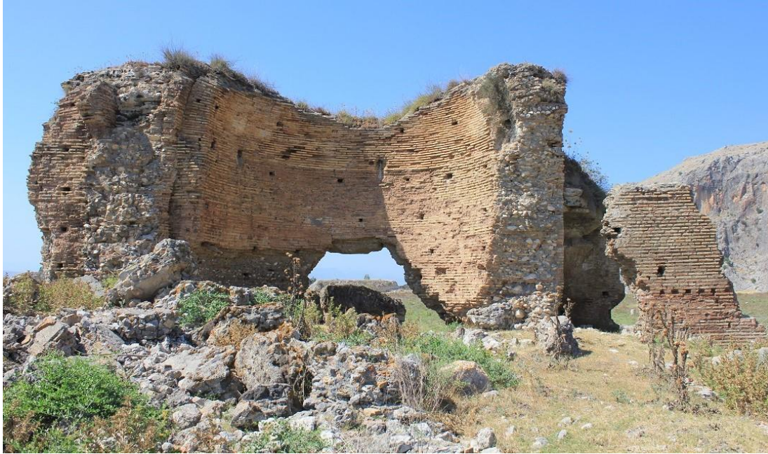
Figure 37: View of the Northern Baths at Anazarbos, showing use of brick-faced mortared rubble masonry, and brick intrados of vaulting, above which was mortared rubble packing using scoria as caementa (photo by author).
