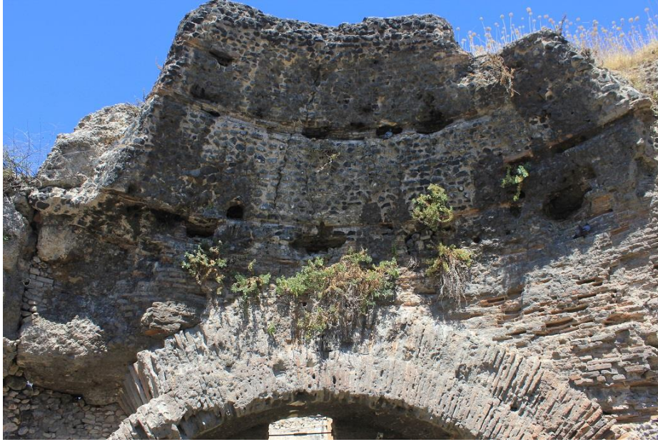
Figure 149: View of the semi-dome in the baths at Tarsus, showing the use of volcanic scoria as caementa and the horizontal division of the mortared rubble by layers of brick (photo by author).
