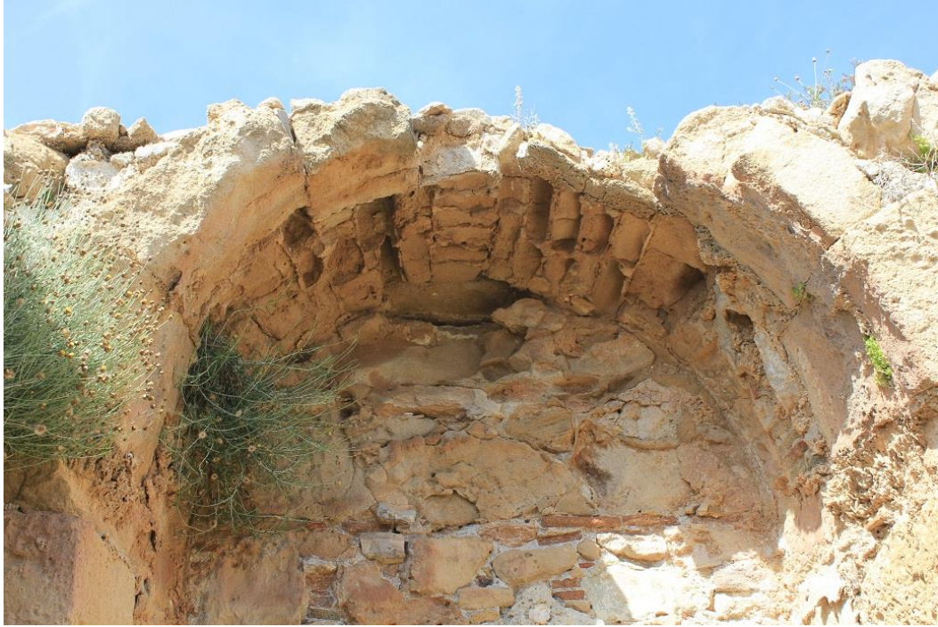
Figure 155: Close-up view of small vault in the baths at Ayios Georgios of Peyeia built of small cut blocks of sandstone laid radially with mortar (photo by author).
