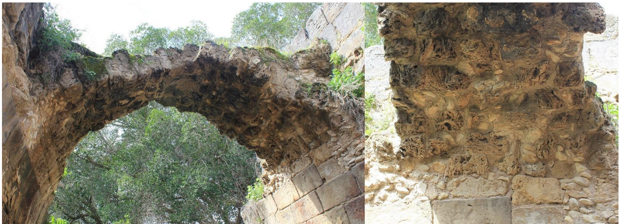
Figure 160: Remains of vaulting in baths at Hammat Gader, showing construction from light-weight tufa set in mortar (photo by author).
