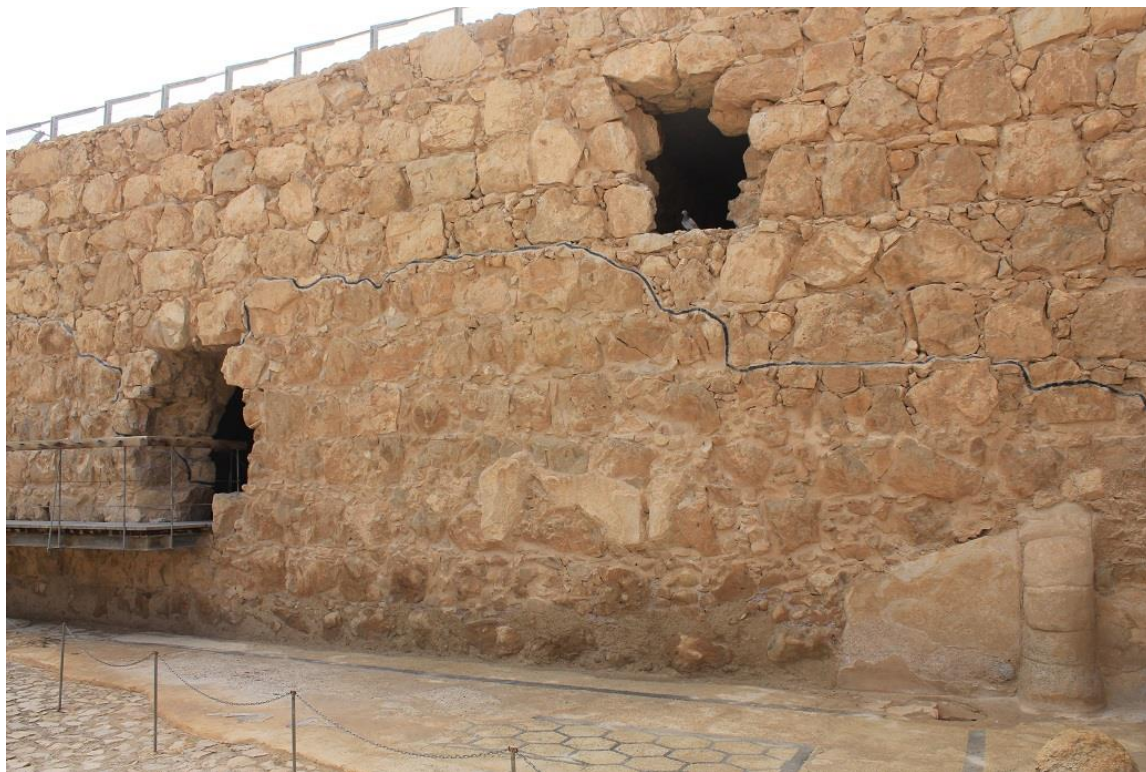
Figure 107: View of thermal block of the Large Baths at Masada, from the north, showing masonry of roughly worked local dolomite with small cobbles as chinking stones (masonry beneath black line is original) (photo by author).
