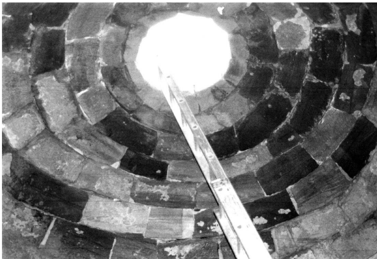
Figure 173: Close-up view of the oculus of the northern dome in the misidentified “baths” near the Temenos Gate in Petra (Rababeh 2005, fig. 6.19a).
