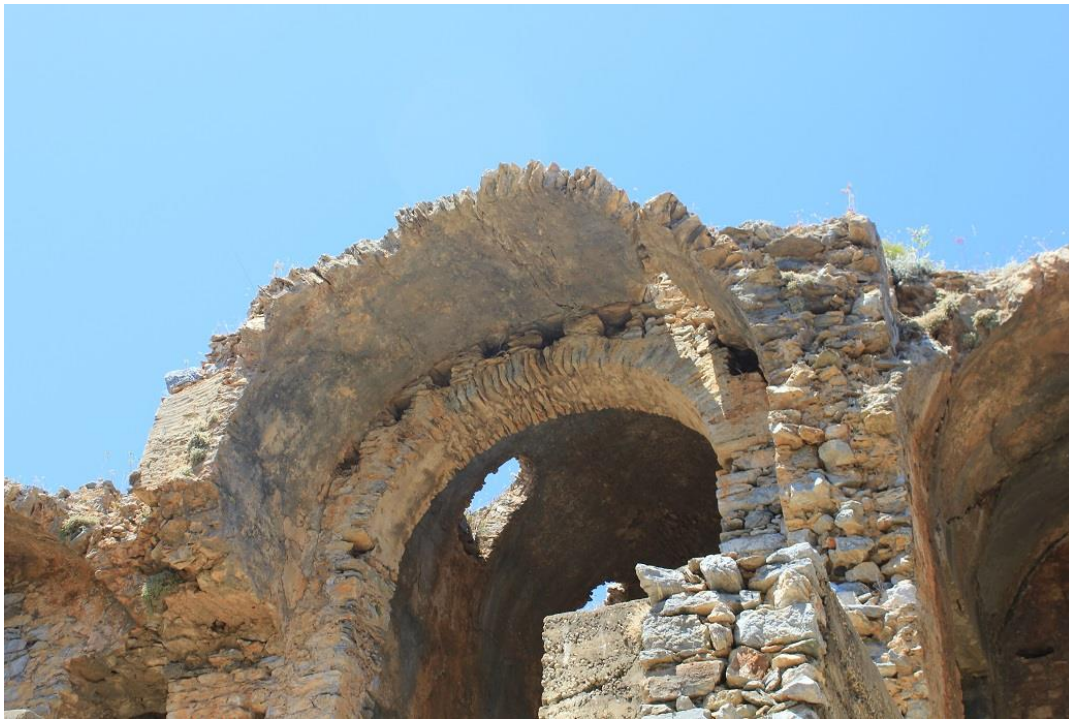
Figure 146: Close-up view of vaulting of Bath II 7 A at Anemurium, from northeast, showing use of irregular limestone blocks set radially (photo by author).
