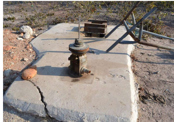
Figure 3.4: Image of a borehole pumping station (Nandjato, 2017)
