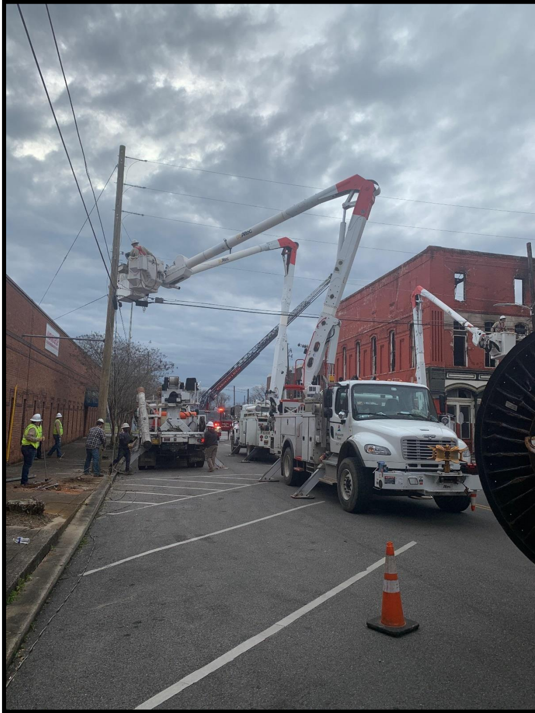
Figure 5. Multiple aerial approaches involving water and power lines were employed. Photo by W. E. Arlinghaus.
