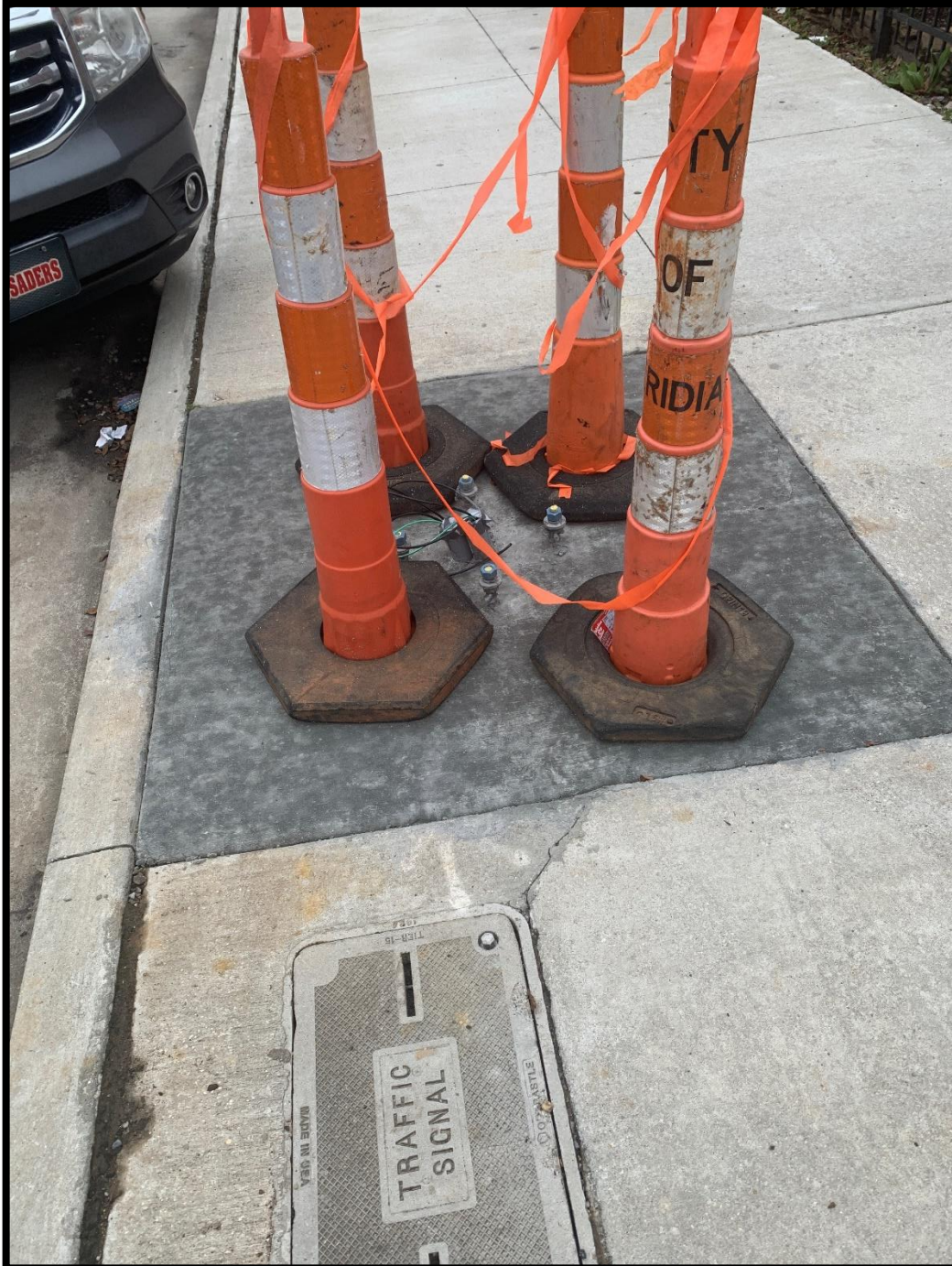
Figure 6a. New pad for streetlight near the Brickhaus and Courtyard. Photo by W. E. Arlinghaus.
