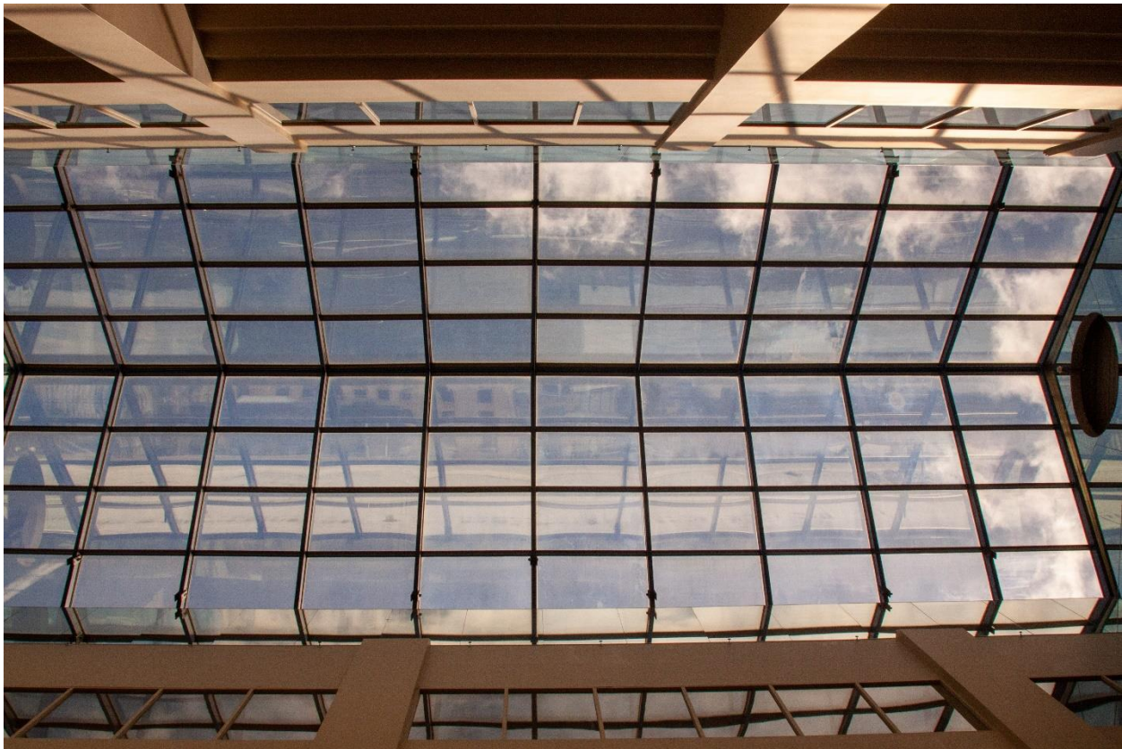
Fig. 6. A photograph of the skylight within the station's lobby: Hudson, Craig. 25 April 2021.
