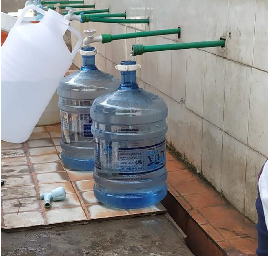
Fig 2: Taps at a water filtration plant in Lahore, Pakistan. The broken head of the tap can be seen on the floor tile.
