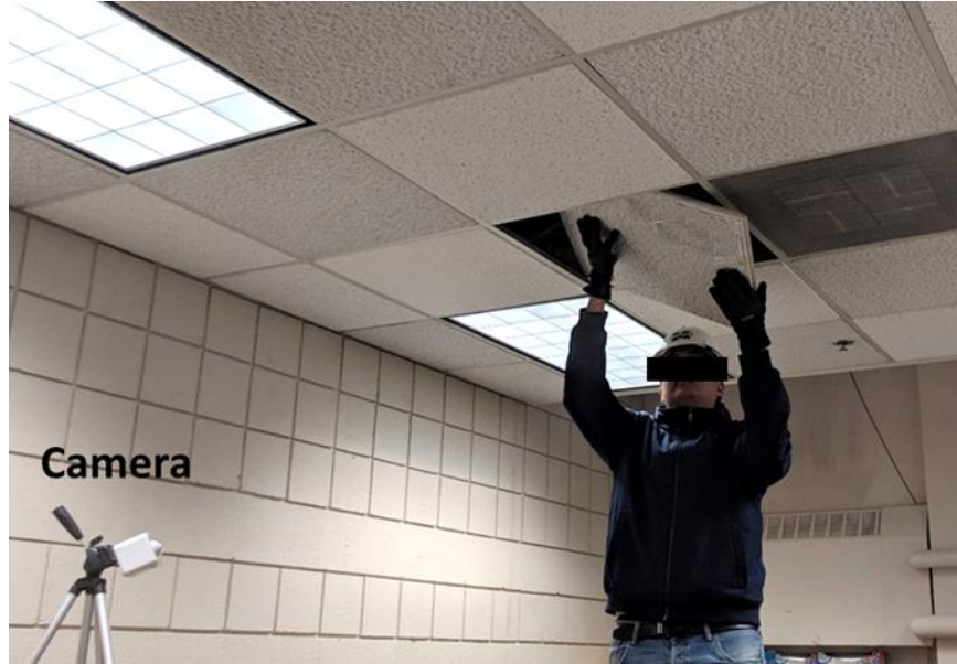
Figure 3.21 Ceiling Tile Installation Demonstration Video Collected in the Laboratory with an Iso View Camera.
