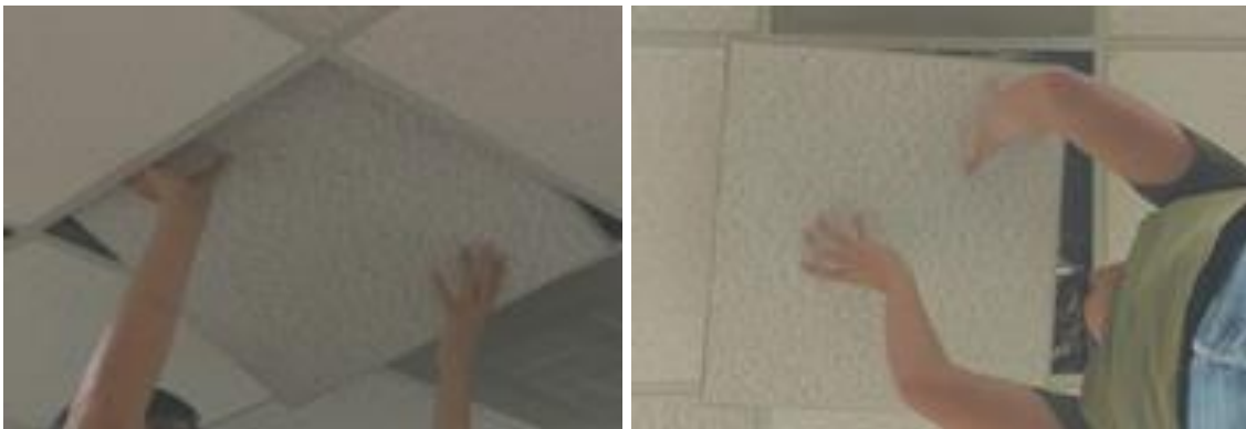
Figure 3.22 Example of the Ceiling Tile Installation Demonstration Video with Two Different Camera Viewpoints (Iso View and Bottom View).
