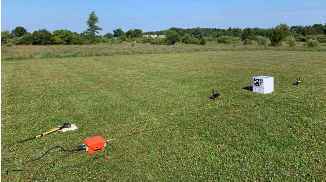
Figure 4-8. SASW field tests for comparison of data acquisition from UAV-deployed wireless geophones and a commercial wired system.
