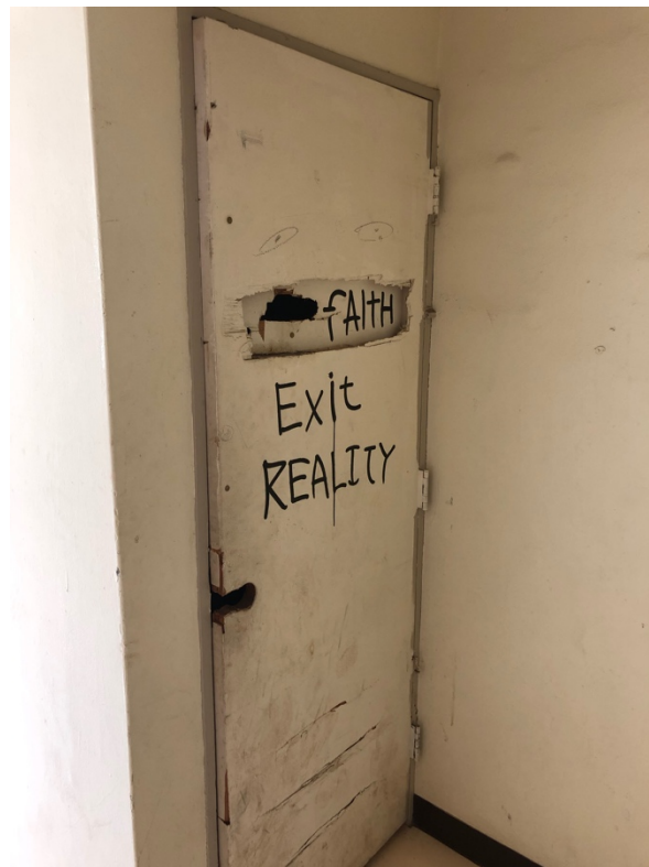
Figure 10: The broken door with messages
