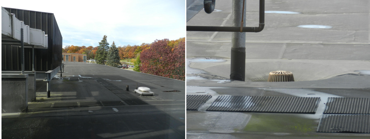
Figure 9. Sample photographs of flat roofs and internal drainage system above the Herbert H. Dow Building (Photos by Arthur Yang). Water can be seen pooling in the background of the right picture, behind the internal drain opening.
