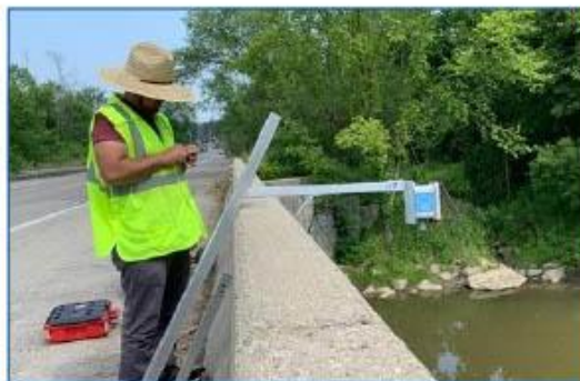
Figure 7. UM student servicing sensor node Source: UM Project Team
