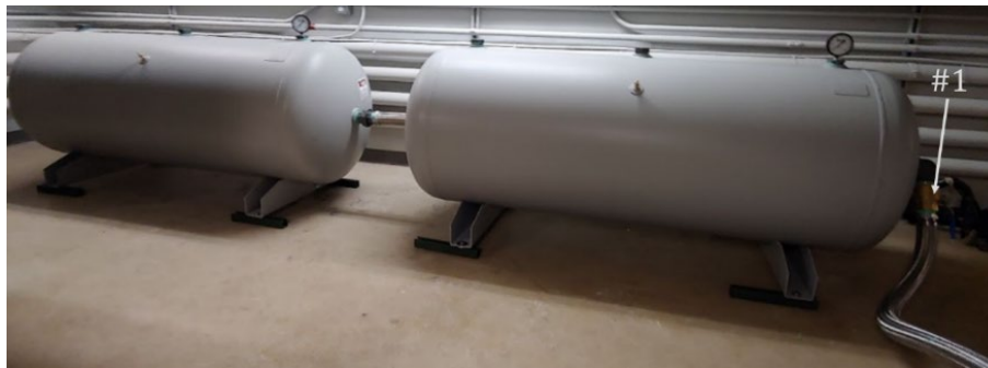
Fig. 5.17. Assembled receiver tanks.
