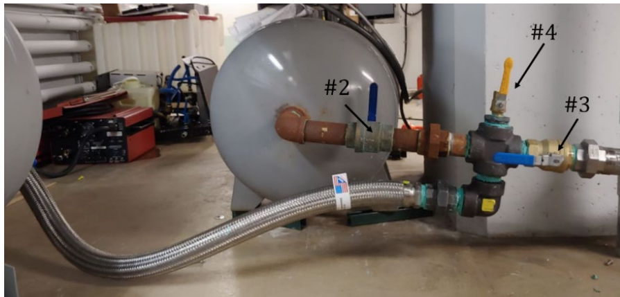
Fig. 5.18. Pneumatic cross intersection from air compressor to remainder of the system.
