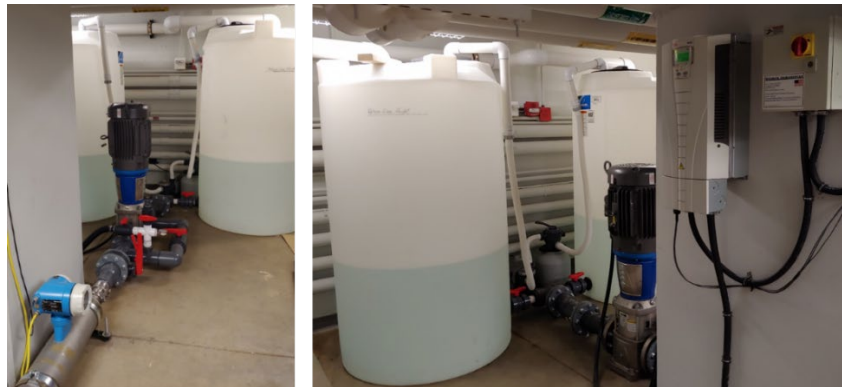
Fig. 5.14. Assembled liquid circulation system.
