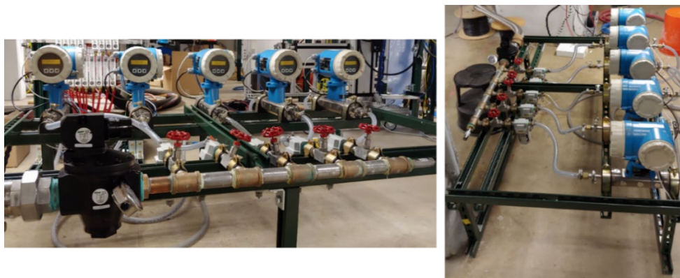
Fig. 5.20. Pressure regulator connected to the manifold system where the flow is split into five gas lines.
