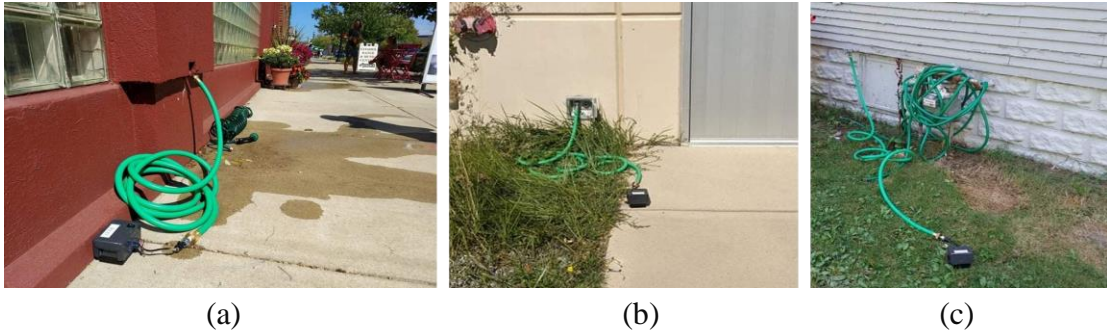
Figure 3-6. Photos of 3 sample installations out of the 9 selected locations that were monitored using water pressure sensors.
