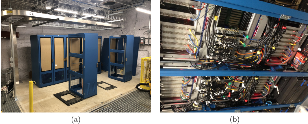
Figure 2.9: Electronics racks which house the DAQ system of LZ, during installation ( left ) and post installation ( right ).
