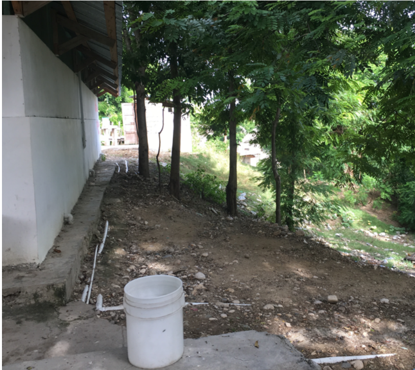
Figure 5-3: The side of the CTC (cholera treatment center) in Mibalè, where exposed and cracked PVC drainpipes are just some of the traces of its disrepair. Photo by author, 2017.
