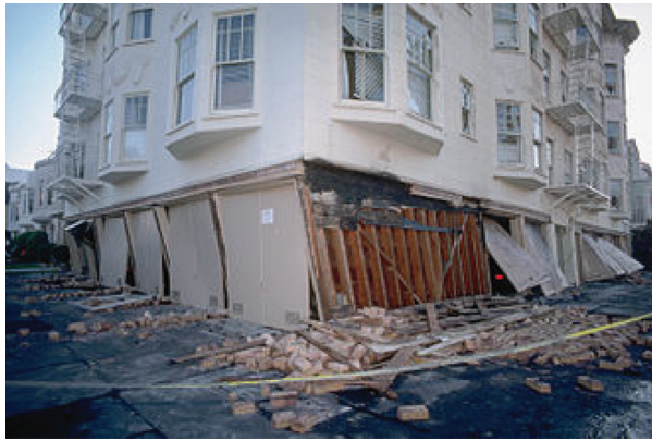
(A) Observation of soft-story collapse during the Loma Prieta earthquake (J.K. Nakata, U.S. Geological Survey)
