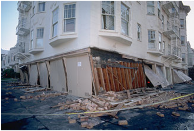
(a) Observation of soft-story collapse during the Loma Prieta earthquake (J.K. Nakata, U.S. Geological Survey)
