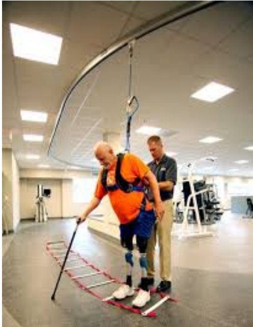
Figure 2. Ceiling-mounted track system for physical therapy
