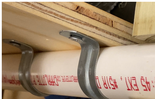
Figure 29. Bracket screw loosened from initial position after 200 lbs testing.
