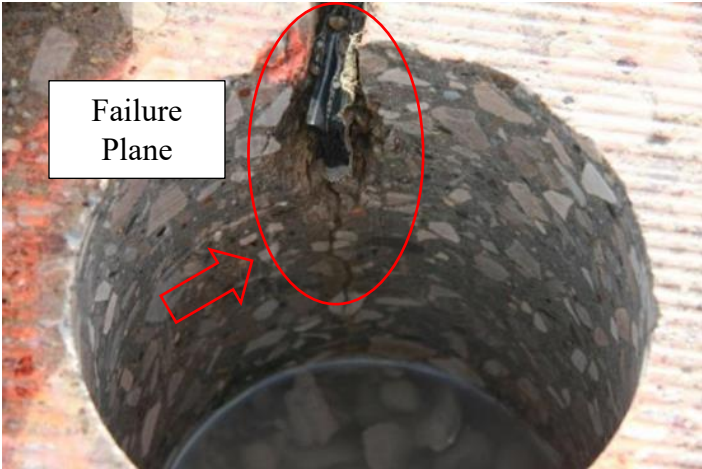
Figure 1.2 Joint core showing erosion of the cementitious binder (courtesy of Prof. Will Hansen)
