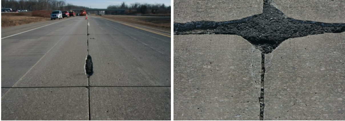
Figure 1.1 Joint spalling in JPCP on M-14, Ann Arbor, Michigan (courtesy of Prof. Will Hansen)
