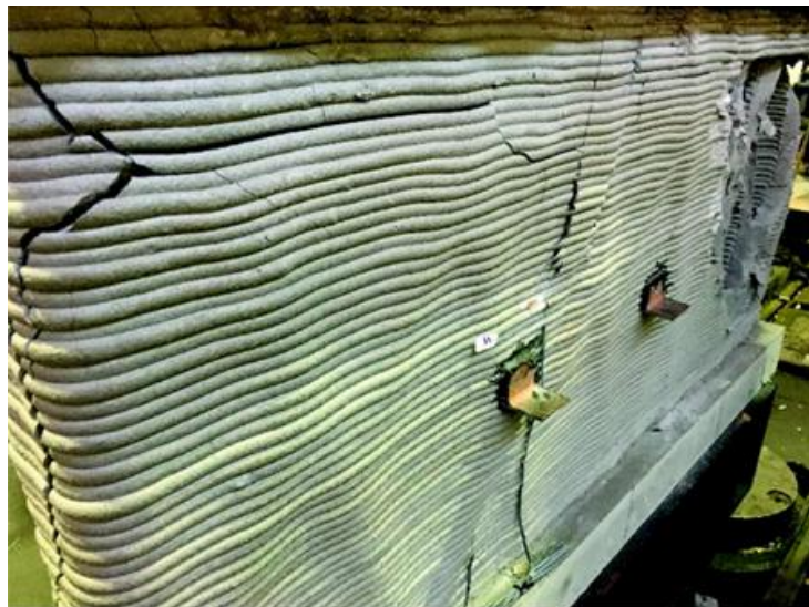
Figure 6.4: Crack pattern of a printed hollow concrete wall under compression (adapted from [149])
