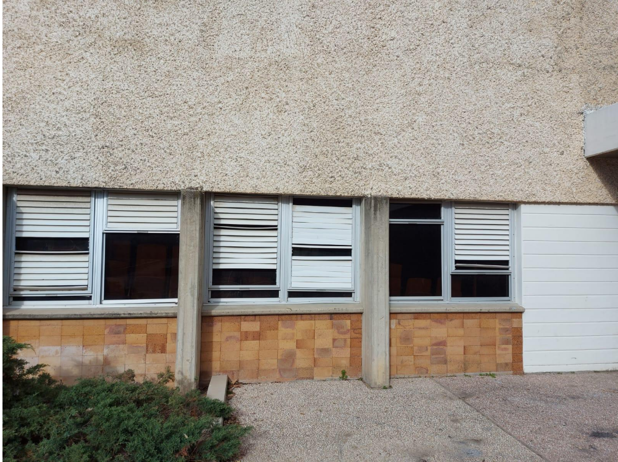
Figure 10 Broken shades in Asif's communal dining hall. Photograph: Omri Senderowicz, 2020.
