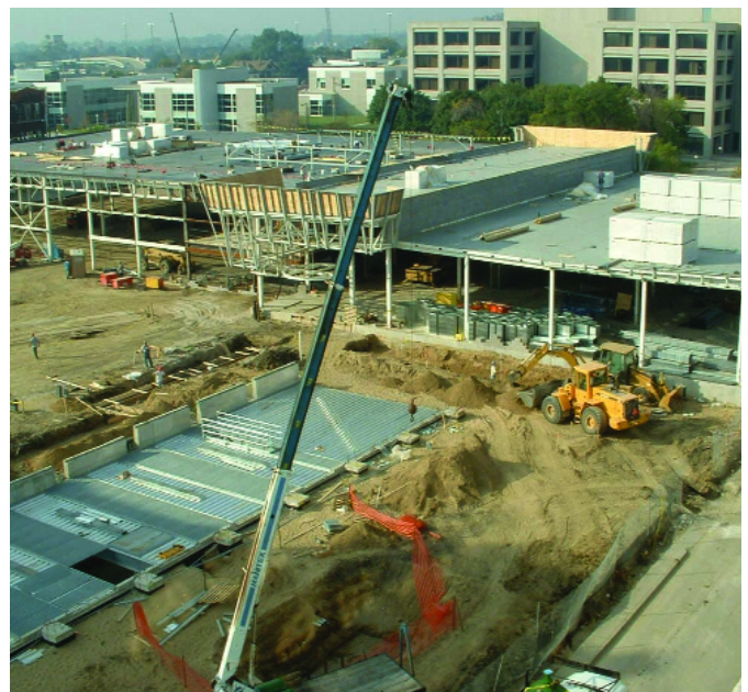
The NextEnergy Center and Microgrid Power Pavilion under construction in Detroit, Michigan
