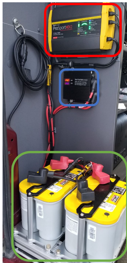
Fig 4-9 Onboard Auxiliary Power System, including (a) 2x Auxiliary high-capacity batteries (green box), (b) an automatic battery isolation system (blue box), and (c) external battery charging system (red box)
