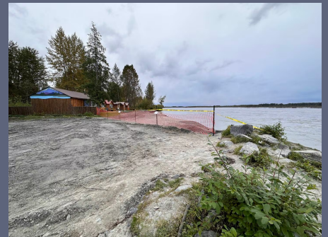
Figure 60. Hinman, S. (2023). The Susitna River has eroded nearly 80 feet into the bank at Talkeetna, officials say. The Matanuska-Susitna Borough on Tuesday declared a local emergency for erosion-related flooding. Anchorage Daily News.
