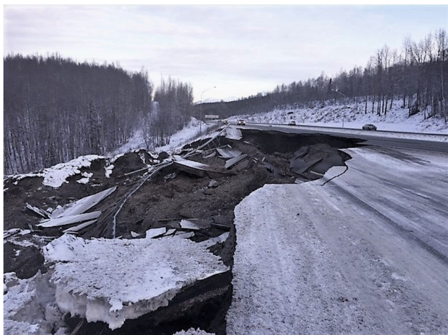
Figure 7. Alaska DOT&PF. (2018). Earthquake Glenn Highway, Mirror Lake. Flickr.
