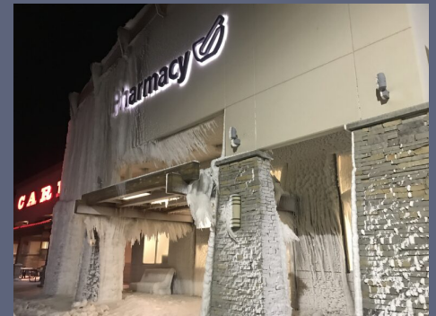
Figure 65. Walker, H. (2022). The Carrs grocery store in Palmer on Monday. Pipes broke and a portion of the roof is gone. Alaska Public Media.
