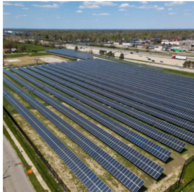
Figure 1.10: Installed solar farm in Sunken Meadow State Park in Kings Park (Suffolk County, easternmost portion of Long Island)
