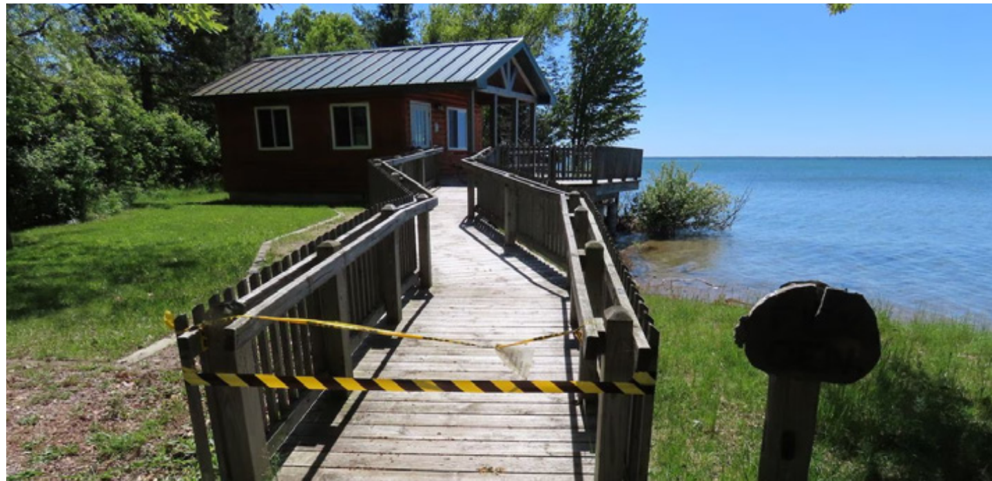
Figure 2.17 Eroding Shoreline Close Cabins at Tawas State Park
