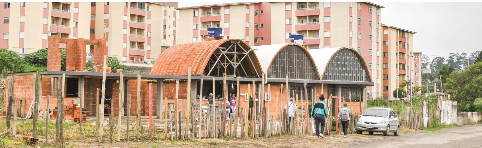
Figure 06.6 Mutirões Dorothy Stang, Jerônimo Alves e Martin Luther King Project site, looking north towards the beginning stages of construction of the project. The small-scale arched buildings pictured will be the commercial portion of the project. The buildings in the background of this image are part of a separate neighboring project.
