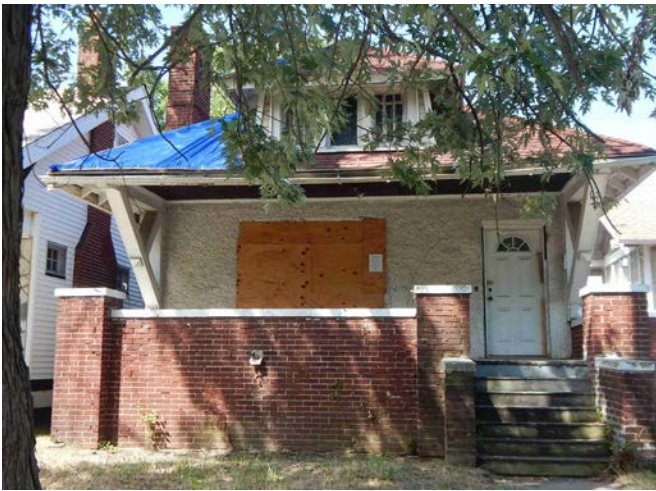
Figure 5.3: Auction House near Nardin Park, Estimated Rehab Cost $ 46,159 (DLBA, buildingdetroit.org)
