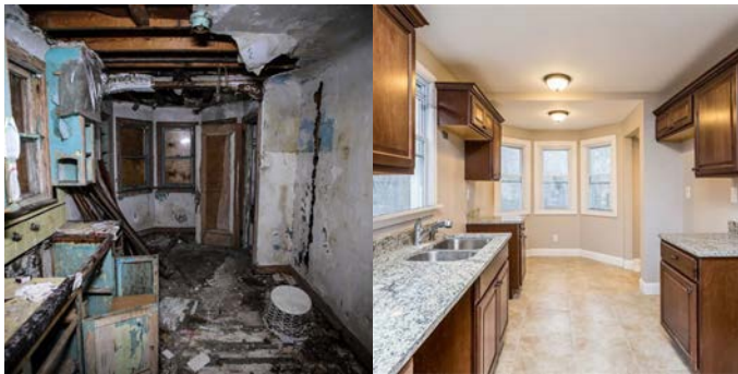
Figure 4.14: Rehabilitation costs alert potential buyers of internal conditions of a DLBA house and the amount of work needed for a home (Paula Gardner, MLive.com)
