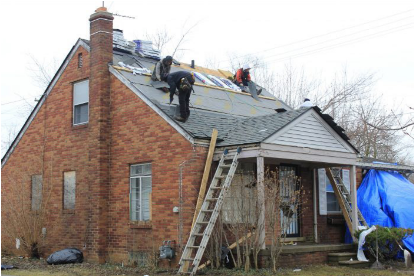
Figure 7.2.5: LifeBUILDERS crew working on a home in Regent Park (TheHUB Detroit, https://www.thehubdetroit.com/housing-and-public-amenity-improvements-coming-to-regent-park-neighborhood/ )
