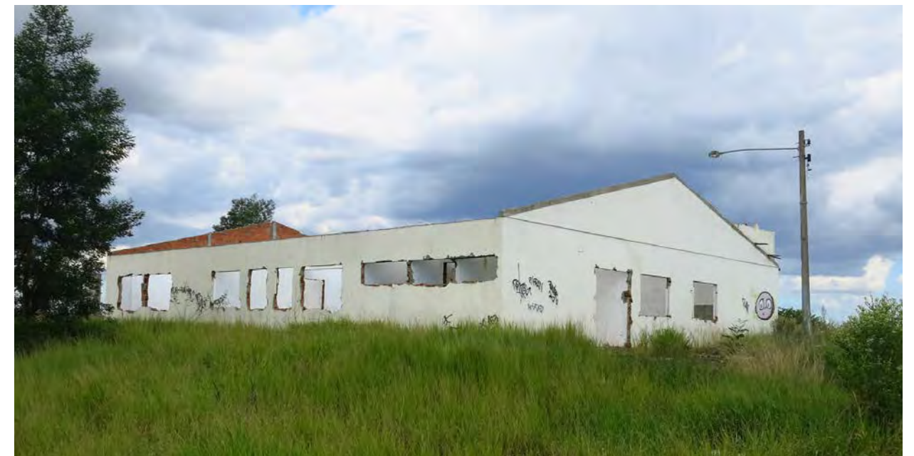
A community center constructed north of Tancredo Neves stands empty after it was scavenged. Located in an unpopulated area, people stripped the building of all reusable material.
