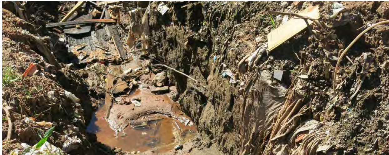
A drainage ditch on the southernmost portion of Santa Marta contains litter, dumped trash, and materials scattered during rainstorm flooding.
