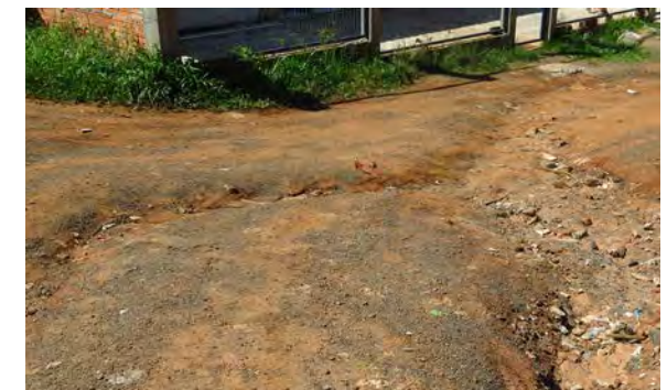
Many unpaved streets are at risk for severe erosion which limit mobility and garbage pickup. Mapping these streets can help the municipality prioritize streets for maintenance.
