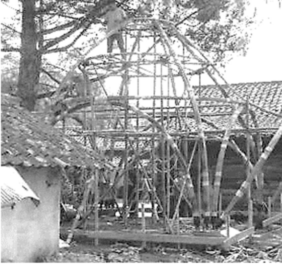
Figure 3. The first project with an arch structural system in bundled bamboo slat construction.
