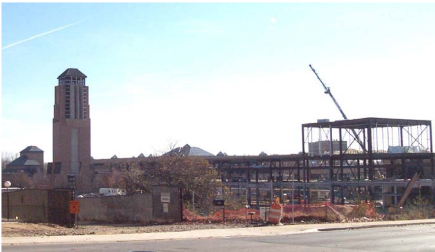
Figure 9. The Walgreen Drama Center is being built on what was a surface parking lot.
