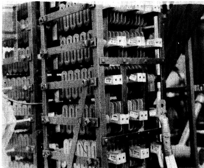
(b) Ballast Resistors, Coil Ballast in Foreground
