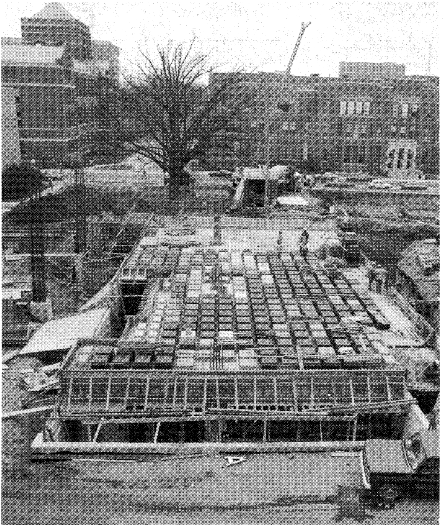
No, this is not a waffle iron. It is the plywood base and fiberglass domes for the first floor concrete slab under the new library. The “waffle” appearance of the floor underside will be the ceilings for the library, classrooms, and office areas.
