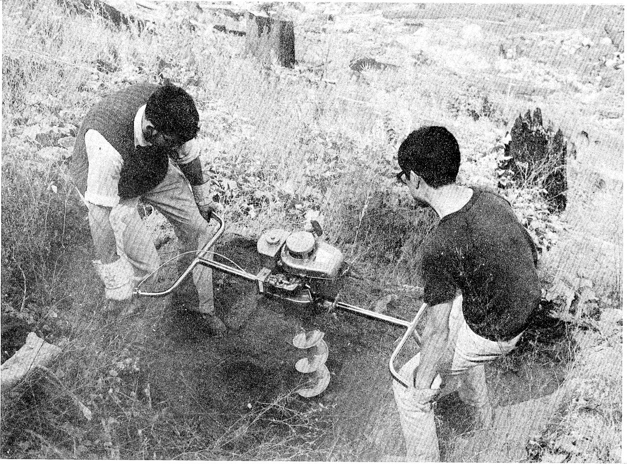
Figure 21. Drilling a hole for slope indicator casing using a portable, power auger.
