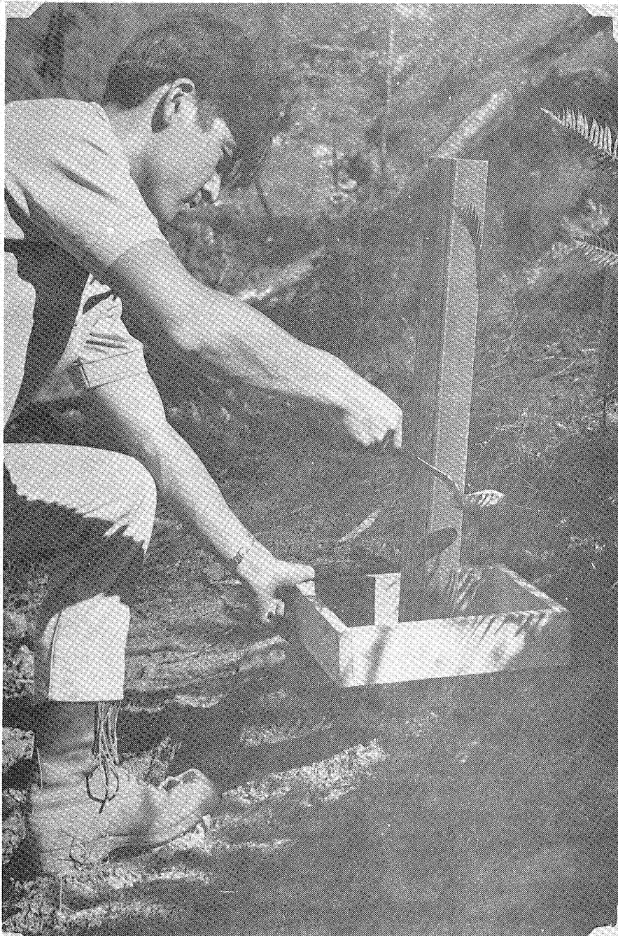
Figure 23. Backfilling around slope indicator casing using the "single grain air dropping" technique.
