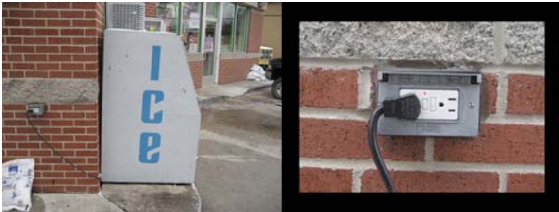
The corner gas station had an icebox on the outside of their building. The outlet around the corner powered it.
