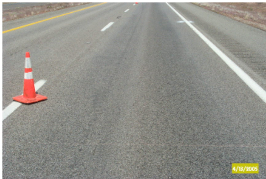
Figure 7. Pavement scuff in the left wheelpath.
