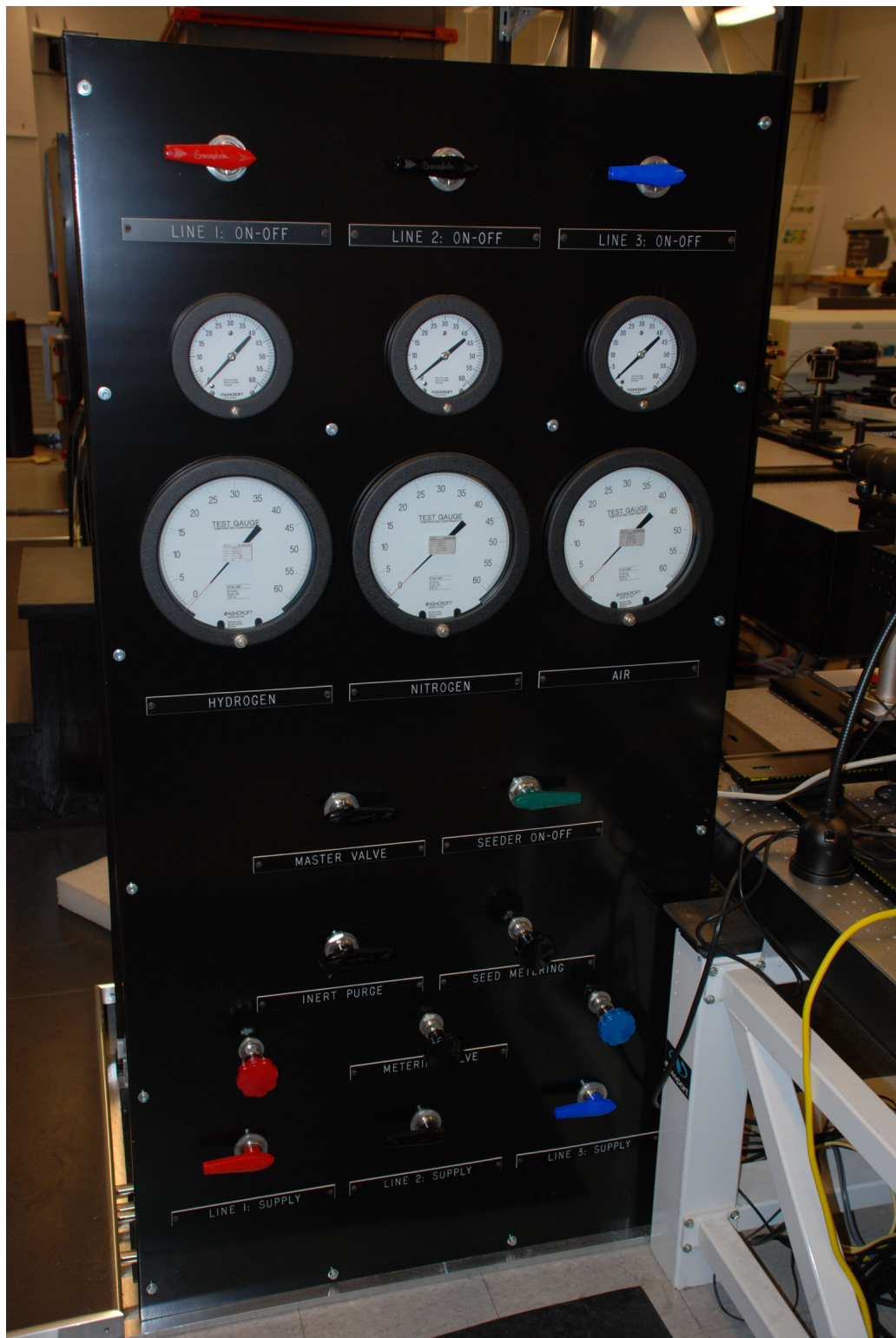
Figure 3.7: Photograph of fuel mixing board. The three independent gas lines are identifiable by vertical alignment of pressure gauge pairs. Fine and coarse flow metering valves are located near bottom of mixing board.
