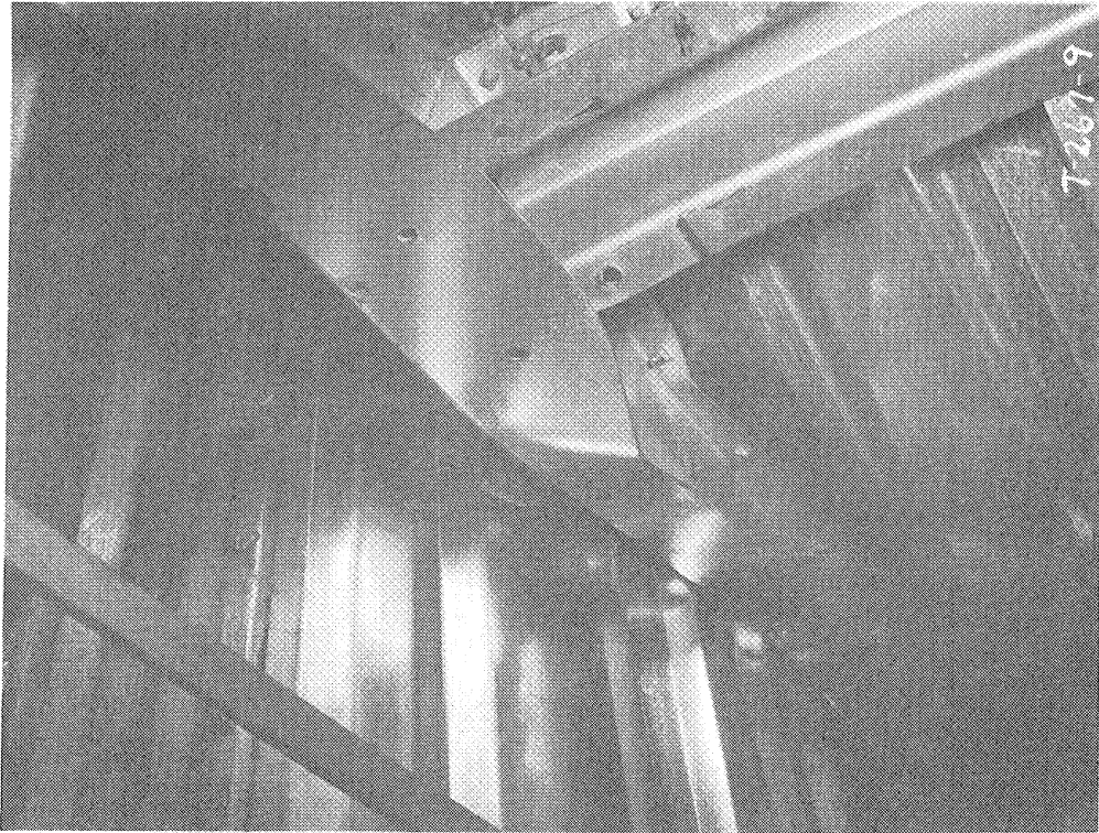
Fig. 2.36—Interior ridge detail at west end of Behlen Building 31.2-b1 after planned test.
