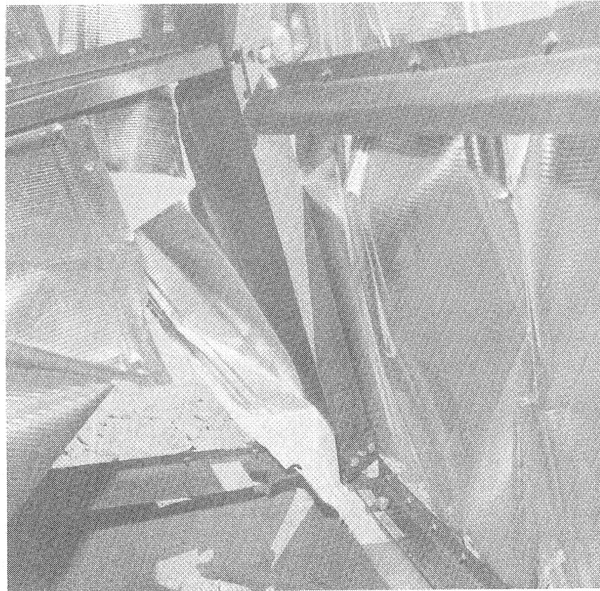
Fig. 2.18—Interior detail of northeast column in Reynolds-Butler Building 31.2-a1 after planned test.
