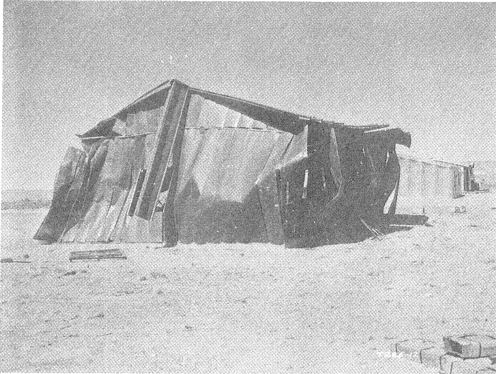
Fig. 2.40 — West end and south side of Armco Building 31.2-d1 after planned test.
