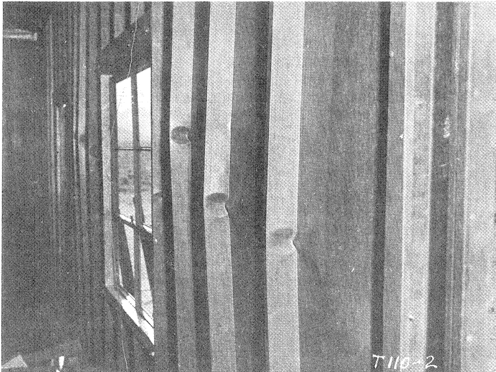
Fig. 2.8—Interior view of damage to north wall of Armco Building 31.2-d1 from unexpected test.
