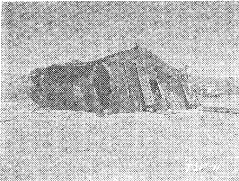
Fig. 2.41 — East end and south side of Armco Building 31.2-d1 after planned test.
