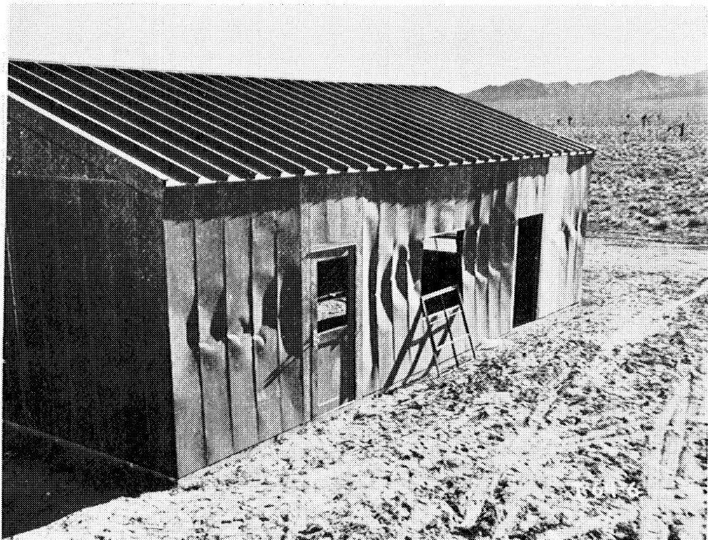
Fig. 2.6—Damage to north walls of Armco Building 31.2-d1 from unexpected test.
