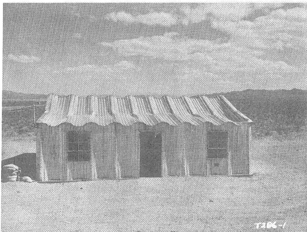
Fig. 2.31—North side of Behlen Building 31.2-b1 after planned test.
