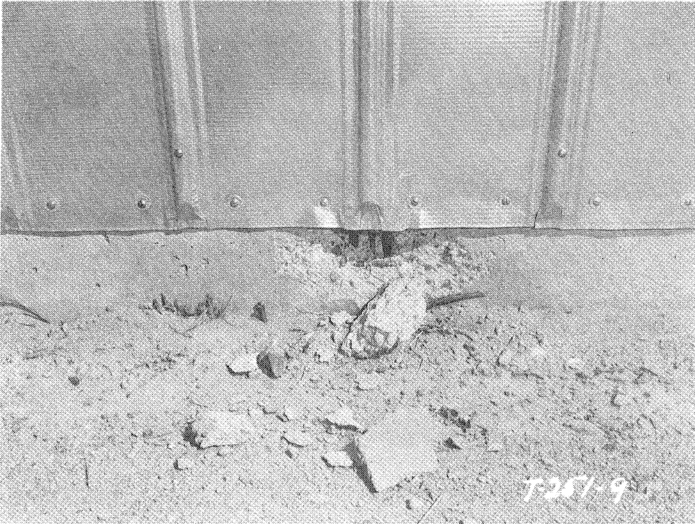
Fig. 2.47—South side of east interior column footing of Reynolds-Butler Building 31.2-a2 after planned test.
