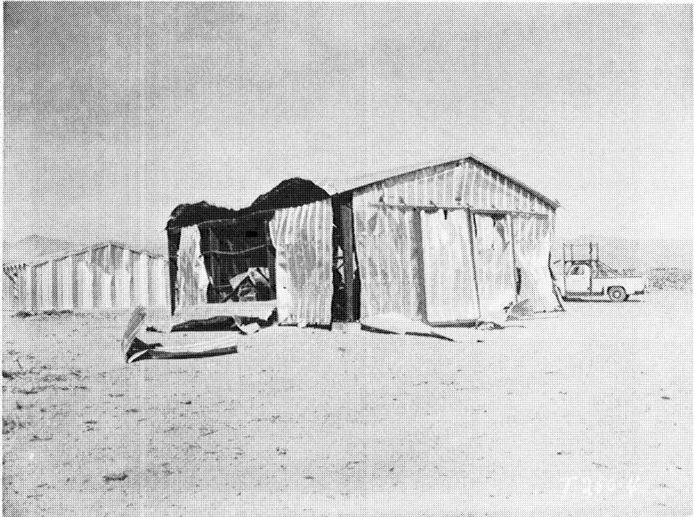
Fig. 2.26 — South side and east end of Reynolds-Butler Building 31.2-a1 after planned test.
