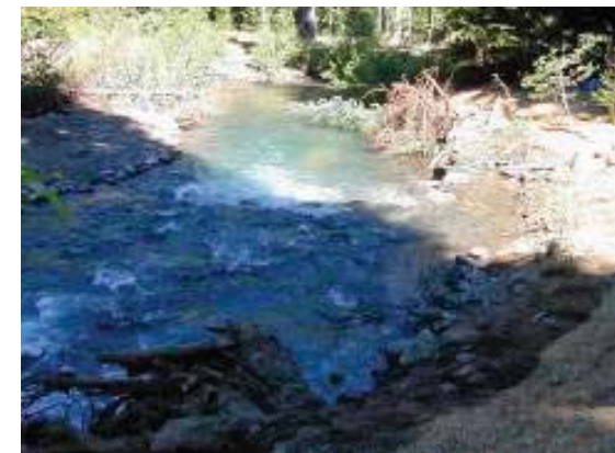
A downstream view of a completed J-Hook vane and the associated root wad and treetop for habitat complexity.
